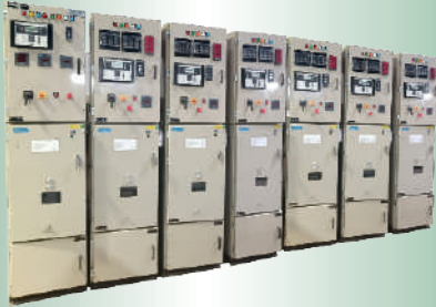
33 / 11 KV, HT Panel
